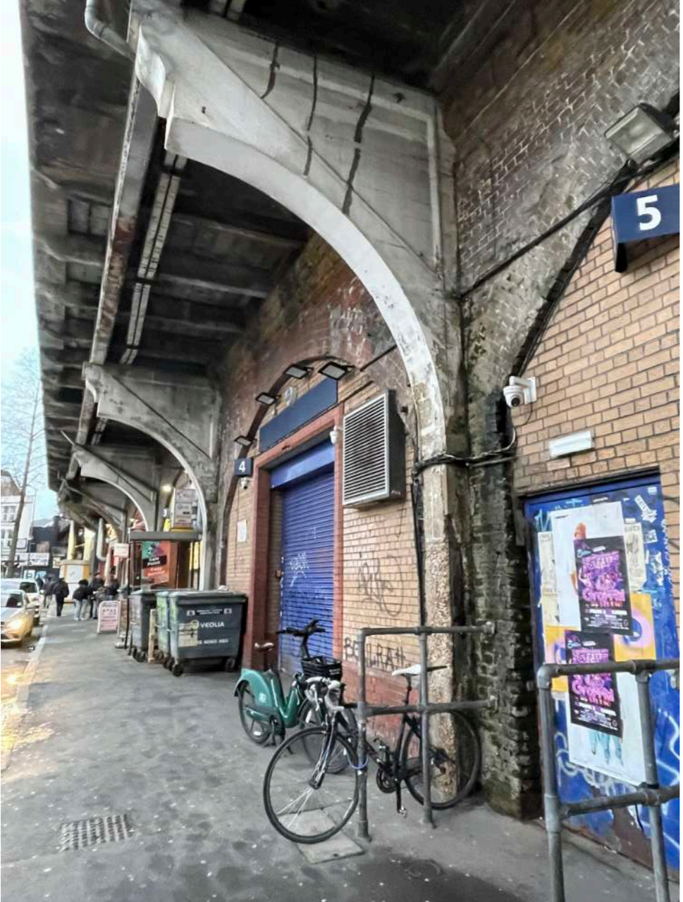
The re-bar at the base of the cast in-situ concrete bracket has become exposed and subject to further weathering and spalling.
